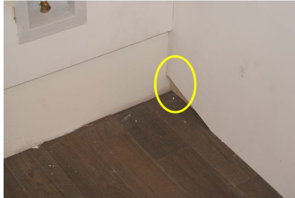
Missing baseboard behind refrigerator.
