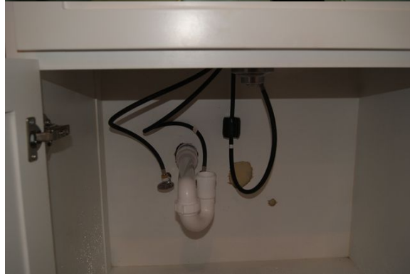
Drain line plumbing was inoperable at multiple sinks at the time of inspection.
