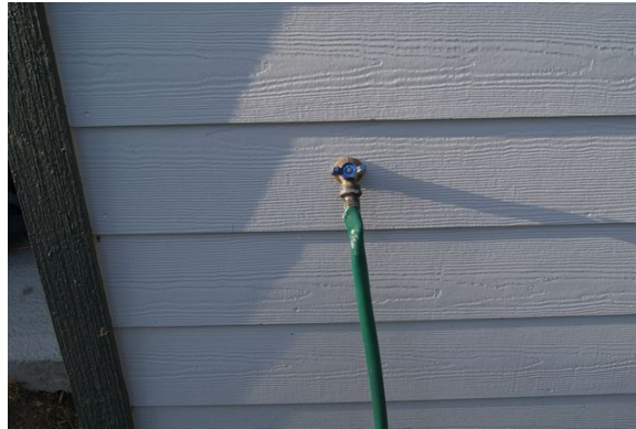
Exterior hose bibs do not have back-flow prevention device.
